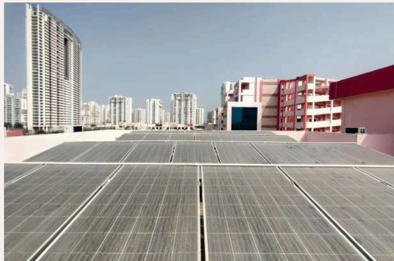
SOLAR PANELS ON ROOF
